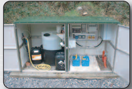
● Kiosk Dosing Station.
